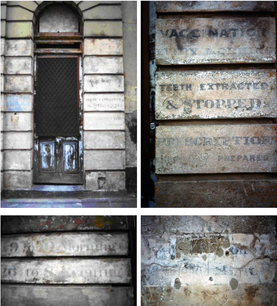
Royal Terrace; original or early signwriting exposed on the Gertrude Street flank. Miles Lewis.
